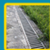
Storm Water Drainage
